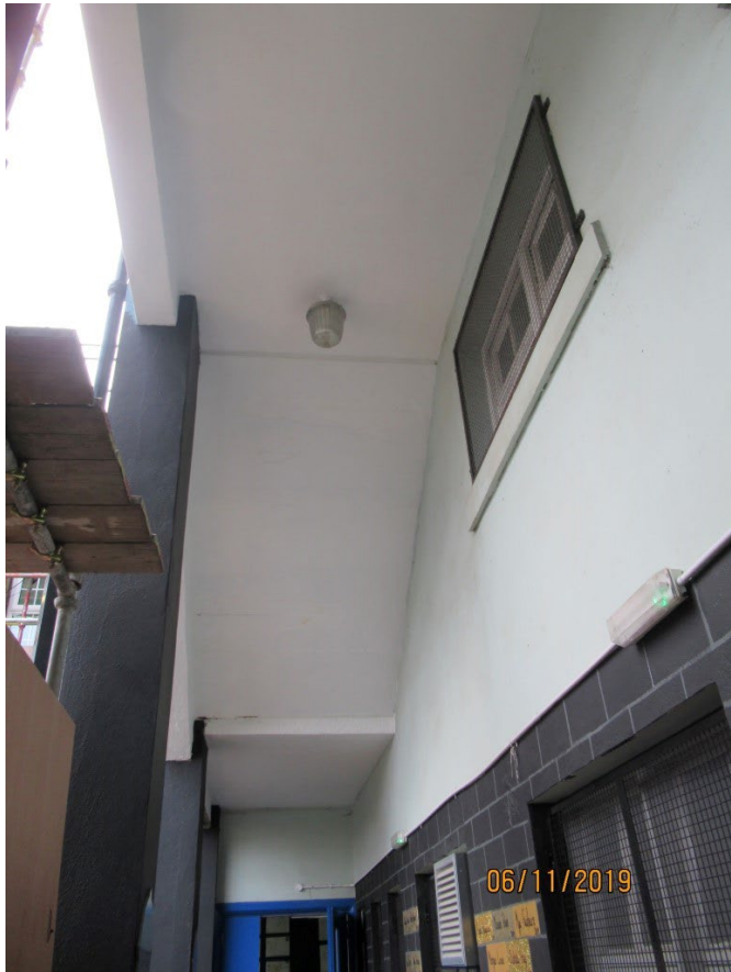
Photograph of Granton Primary School external building fabric & windows after improvements
