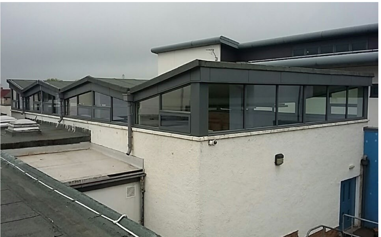
Photographs of windows & cladding at Currie Primary School (Games Hall) after improvements
